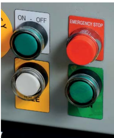
Control Panel Labels
